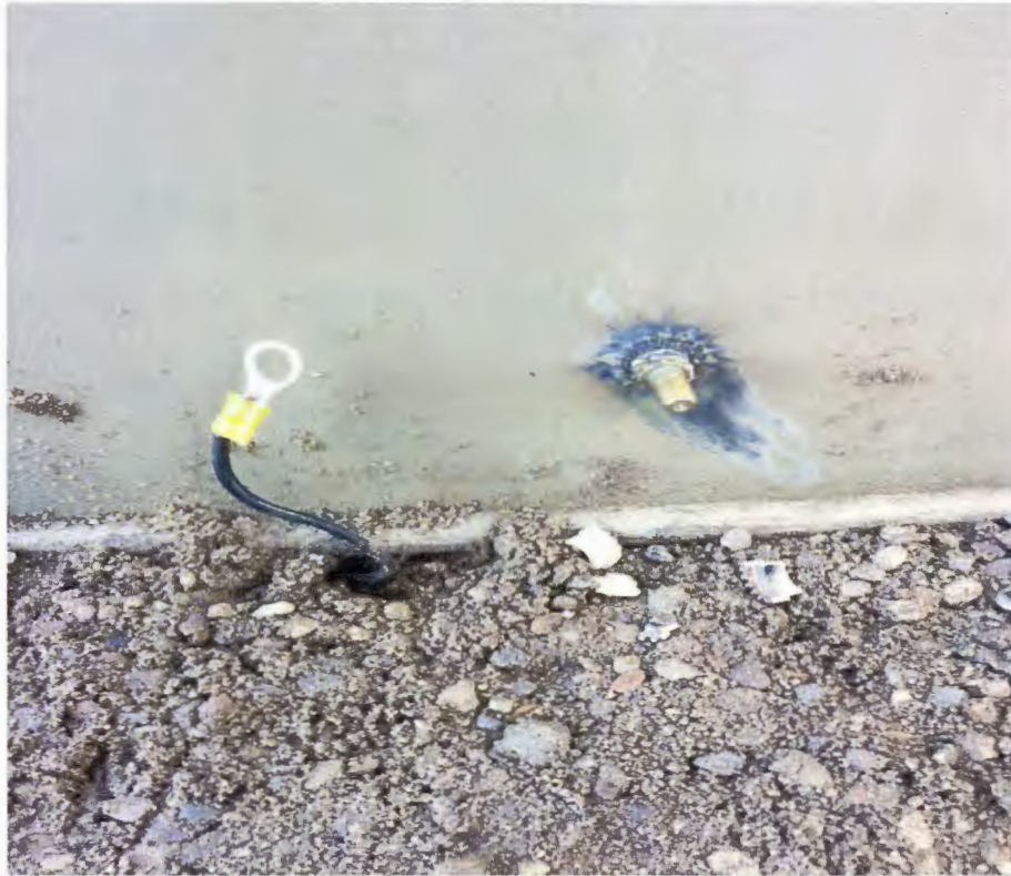
Attachment point brazed to tank
